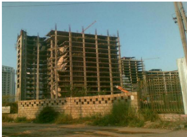
FIG. 1 SHANTINIKETAN TOWNSHIP COLLAPSE
